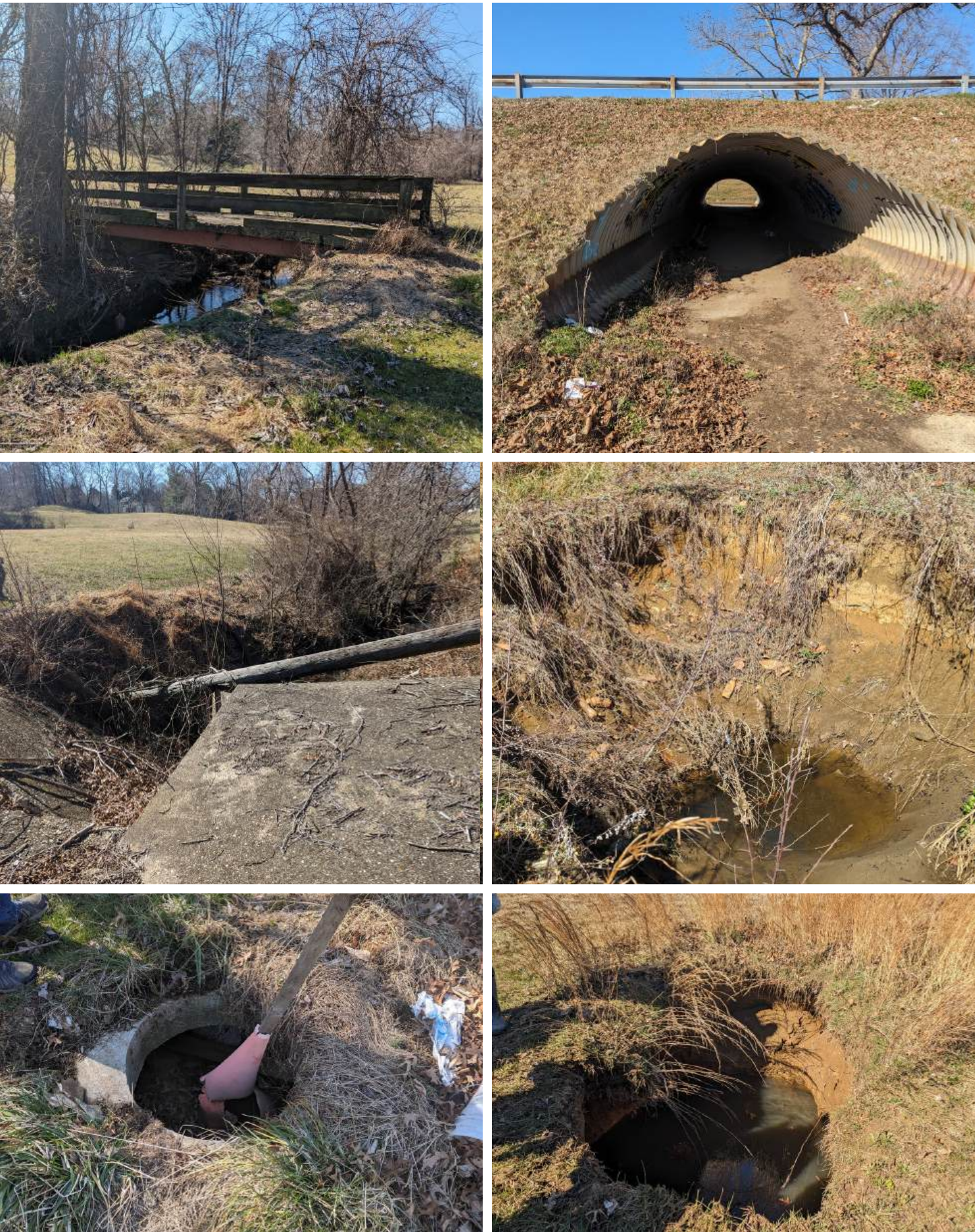
FIGURE 22 Examples of site infrastructure that is failing or in poor condition.
