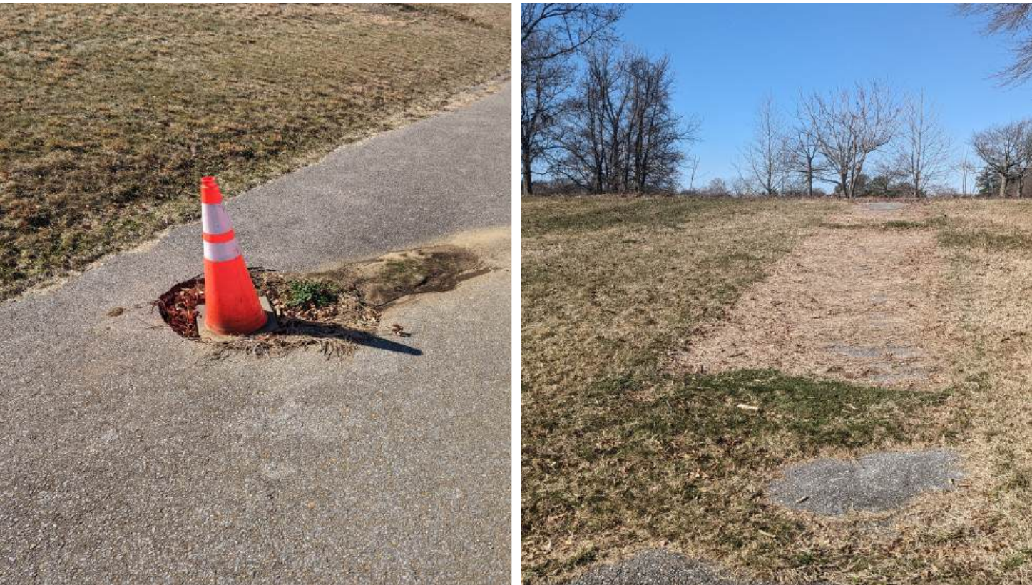
FIGURE 17 Sinkholes and failing pavement illustrate the poor condition of the existing cart path network.
